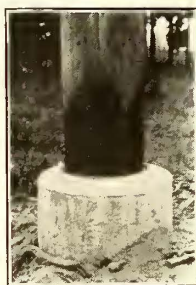
DECAYED POLE WITH CONCRETE BASE APPLIED
