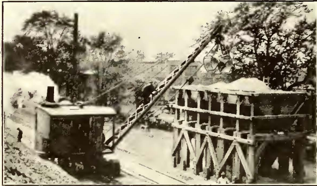
A CRANE AND CLAMSHELL BUCKET AND OVERHEAD BUNKER GREATLY FACILITATE HANDLING OF MATERIALS AND LOADING TRUCKS AT STORAGE YARD
