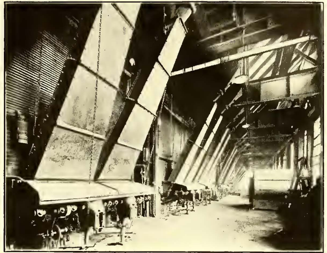
LOOKING DOWN THE BOILER-ROOM FIRING AISLE
