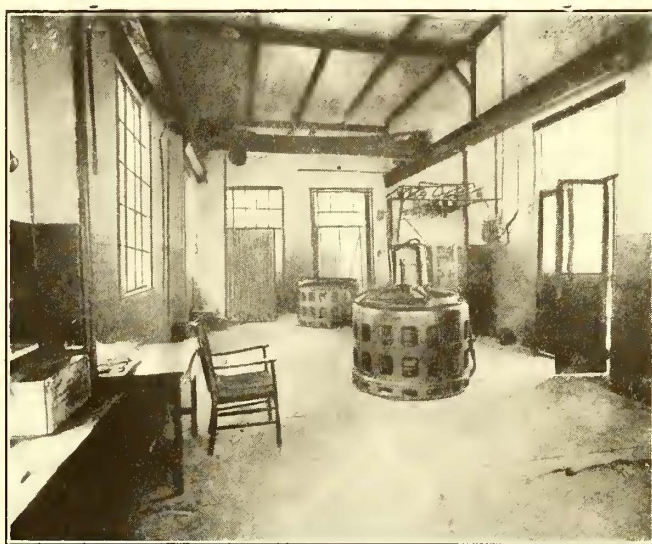
MOTOR ROOM, WITH SWITCHBOARD IN BACKGROUND
