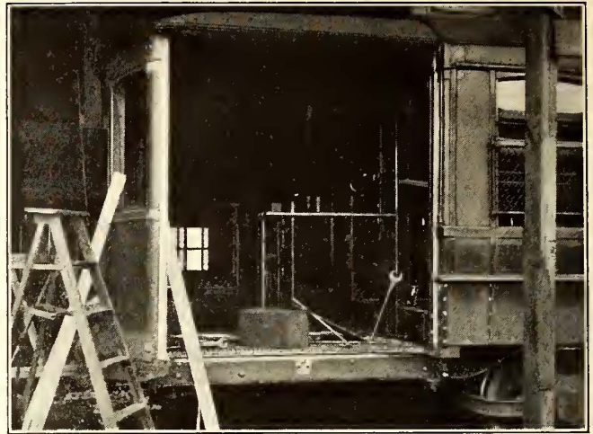
CAR IN THE PROCESS OF CONVERSION. PLATFORM MUST BE CUT AWAY AND SUPPORT BENT TO ALLOW FOR STEPS. CHANGES ARE ALSO NECESSARY IN BULKHEAD DOORS
