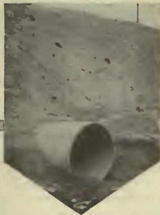
Toncan Metal Culvert under Lake Erie & Northern Ry.
