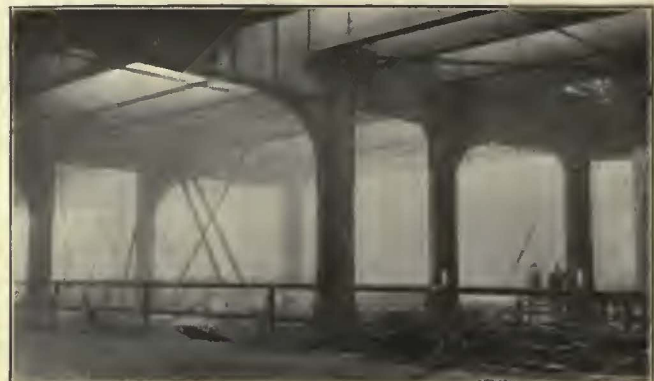
WRECKAGE UNDER THE ELEVATED STRUCTURE
