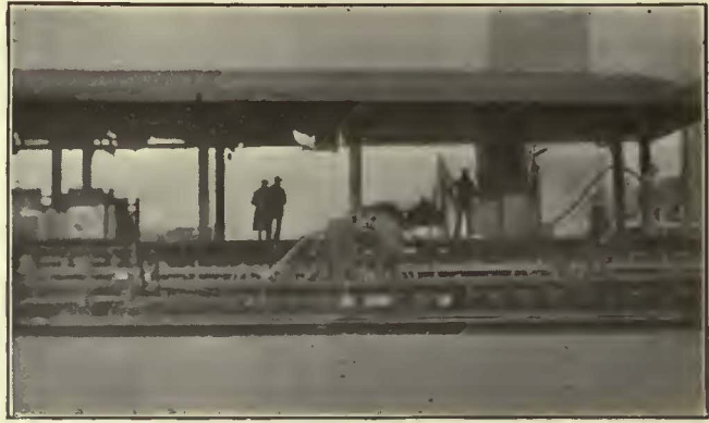
STATION PLATFORM BADLY DAMAGED
