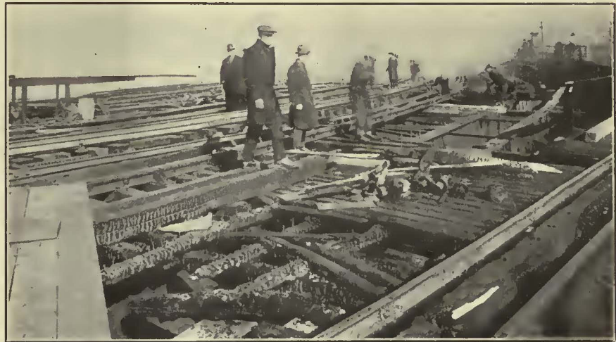
CHARRED TIES AND STRINGERS ON CHICAGO ELEVATED STRUCTURE
