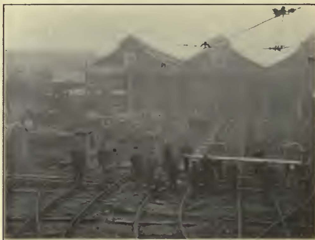
WHERE THE CARHOUSE IS BEING EXTENDED TO CARE FOR THE NEW ELECTRIC EQUIPMENT
