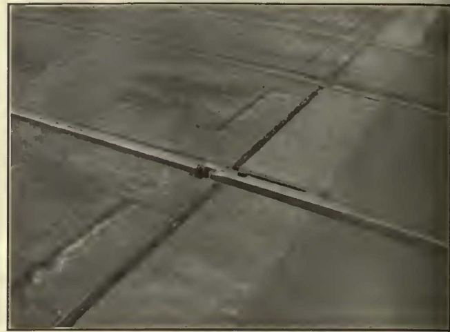
MITERED JOINT IN MANGANESE RUN-OFFS BETWEEN LIFT AND STATIONARY PORTION OF BRIDGE
