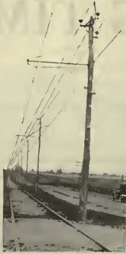
An Outside Plant with 33,000 volt line equipped by the nearby Western Electric Distributing House.
