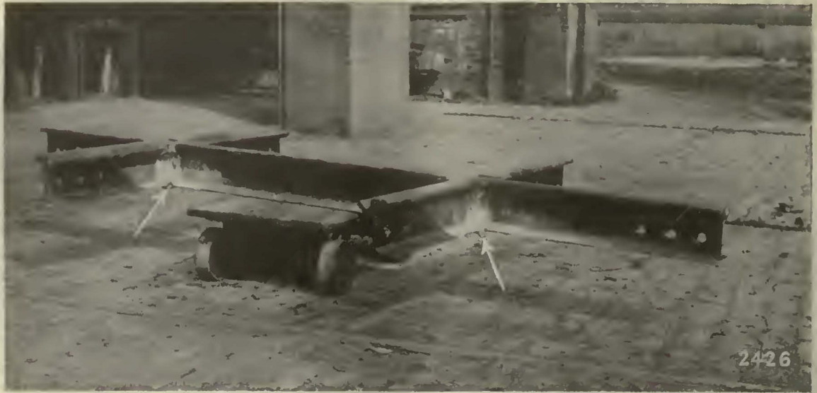
One-half of a single-track crossing constructed by means of Thermit welding for Omaha & Council Bluffs Street Railway, Omaha, Neb.
