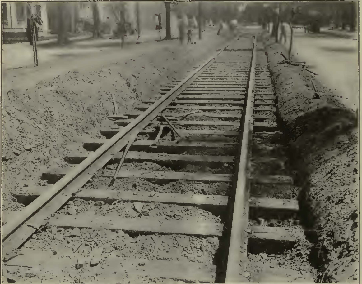
(Recent photograph showing creosoted pine ties supplied by this company in track, New Orleans Street Ry. since 1899)
