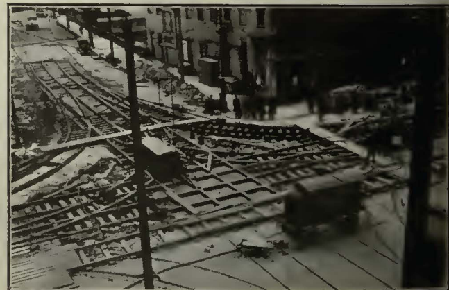
NICKEL CHROME STEEL LAYOUT GOING IN AT EAST WATER AND MICHIGAN STREETS, MILWAUKEE
