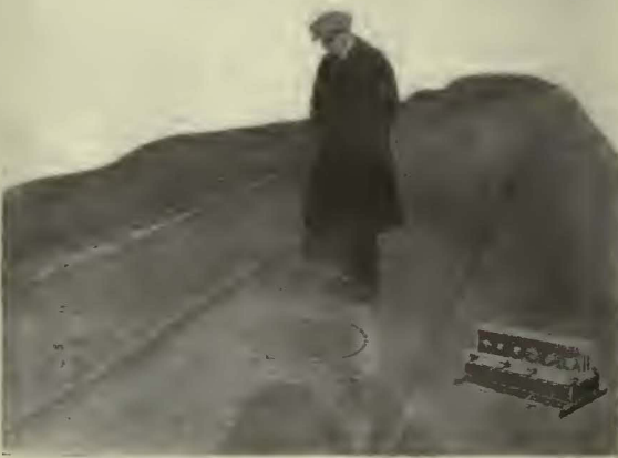
The maintenance on this track by using shims has been enormous and is only short lived. The rails appear to be good, but the joints are battered and low and the constant hammering over them is ruinous to the rolling stock, not to say a word about the lost current. If I could find a cure for this condition at out too great a cost, I believe I could postpone rebuilding this track for six or seven years, and by that time this Company may be in better financial condition.
