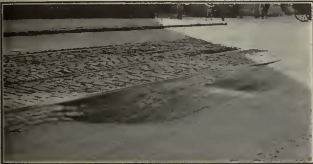
DEPRESSION OCCURRING IN PAVING SURFACE AS A RESULT OF TUNNELING UNDER ROADBED
