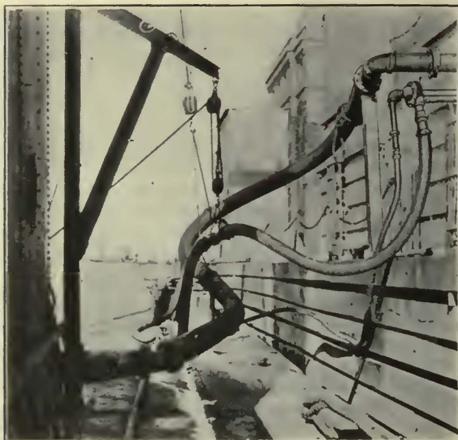
FLEXIBLE OIL AND STEAM CONNECTIONS BETWEEN BARGE AND POWER HOUSE
