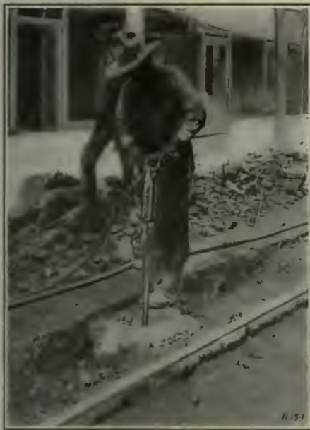
Paving Breakers operated from the Tamper Car show savings up to 75% over handwork.
