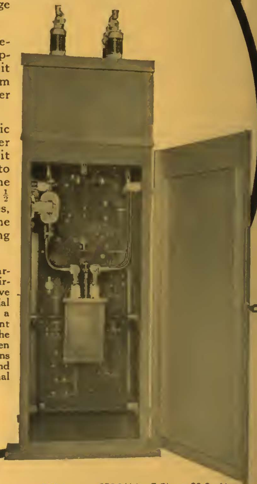
500-Ampere, 2300-Volts, 3-Phase, 60-Cycle Automatic Outdoor Switch House, Periodic Re-closing Feeder Equipment.—Rear View.
