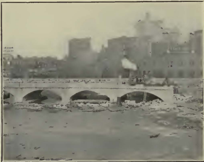
EXTENDING ARCHES OF AQUEDUCT, STREET TO BE ABOVE SUPPORTED ON GRACEFUL SHORT-SPAN ARCHES WITH RAILWAY TRACKS LAID IN THE BED OF THE OLD CANAL. CROSS-SECTION OF COMPLETED STRUCTURE IS SHOWN ON PAGE 908.
