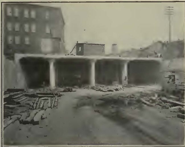
CROSS-SECTION OF SUBWAY AT OAK STREET—AT LEFT, SIDING TO WAREHOUSE ABOVE; NEXT, PASSENGER TRACK; BOTH SIDES OF MIDDLE ROW OF COLUMNS, PLATFORM MAIN STREET STATION; NEXT, PASSENGER TRACK; AT RIGHT, FREIGHT TRACK
