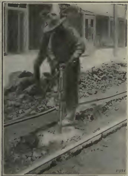
Paving Breakers operated from the Tamper Car show savings up to 75% over handwork.
