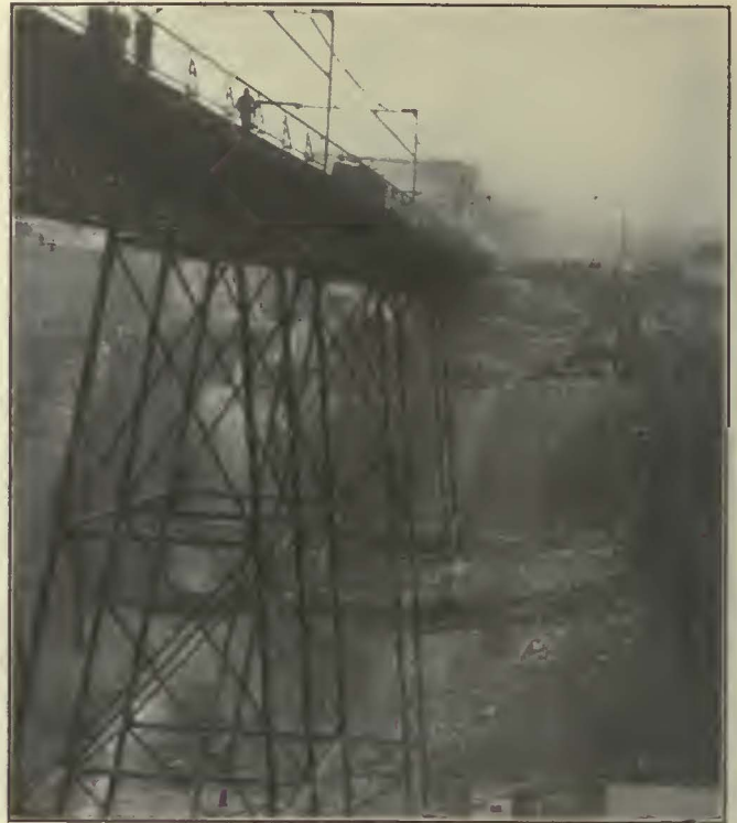
THIS VIEW LOOKING TOWARD THE BELLEVUE SIDE WAS TAKEN AT NOON ON NOV. 25 AFTER THE BRIDGE HAD BEEN MOVED ABOUT 35 FT. THE OLD ABUTMENTS AND CERTAIN RUNWAYS AND JACK SETTINGS ARE CLEARLY SEEN
