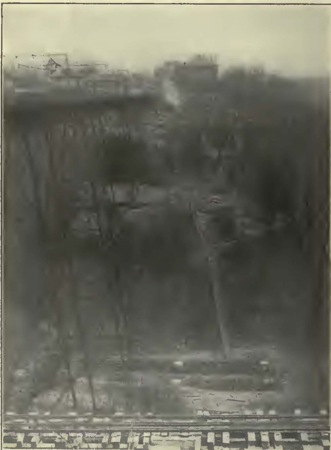
THIS VIEW LOOKING TOWARD THE PITTSBURGH SIDE WAS TAKEN ON NOV. 21 AND SHOWS THE HIGHEST TOWER, NEW TIMBER ABUTMENTS, PEDESTALS, RUNWAYS, ETC.
