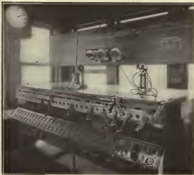
Electro-Pneumatic Interlocking Machine, with Lever Light Indicators and Illuminated Track Model and Clockwork Time Releases
