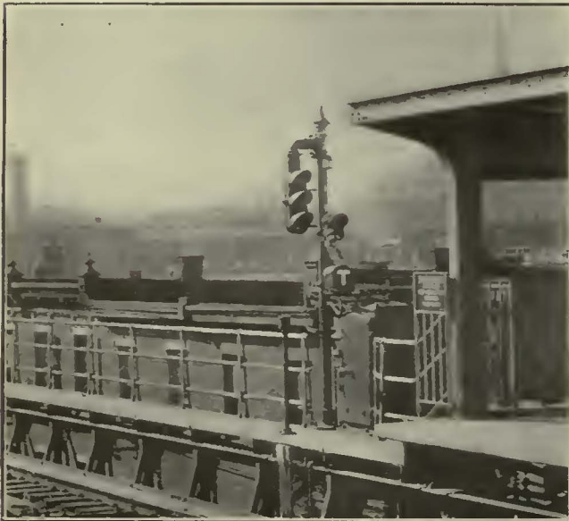
Color-Light Signals at Torresdale Street Electro-Pneumatic Interlocking
