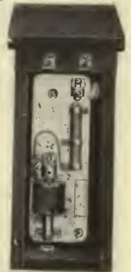
Garton-Daniels D. C. Pole Arrester Door Removed
