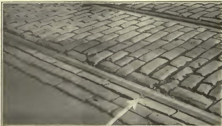
One of many Thermit Rail Welds installed on Shady Ave., Pittsburgh. Still in excellent condition after 10 years' service.
