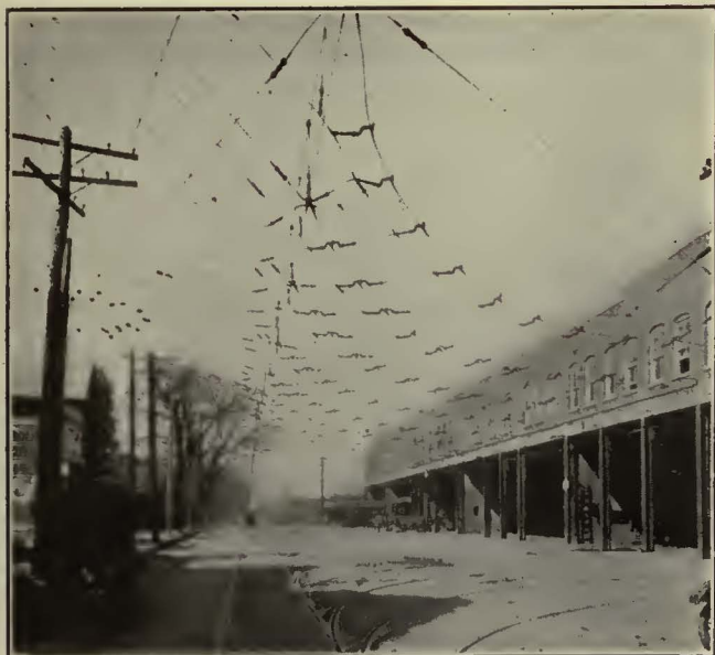
Catenary Messenger Supports and "Back-bone" Reinforcement Insure Durability in the Overhead Network
