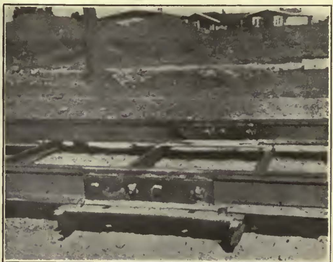
Electrically Welded Joint as Used in San Diego Electric Railway Standard Track Construction
