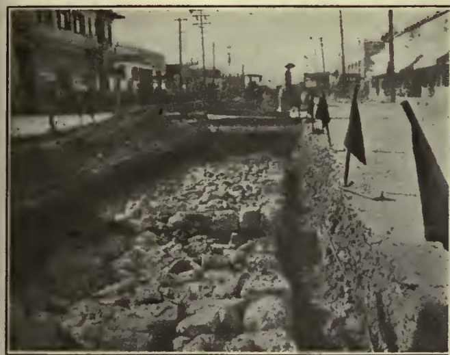
Soft Spot in Adobe Soil, Filled In with Broken Concrete Preparatory to Laying of Track Structure
