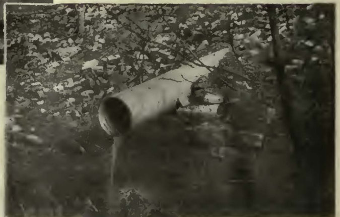
An 18-in. diameter "GENUINE OPEN HEARTH IRON" Culvert Pipe installed under the right-of-way of the C. N. & C. Street Railway Co. at Sunnyside Stop on the Cincinnati-Fort Thomas Line.
