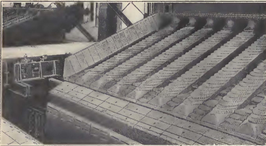
Interior View of Stoker Showing Ash Discharge Device
