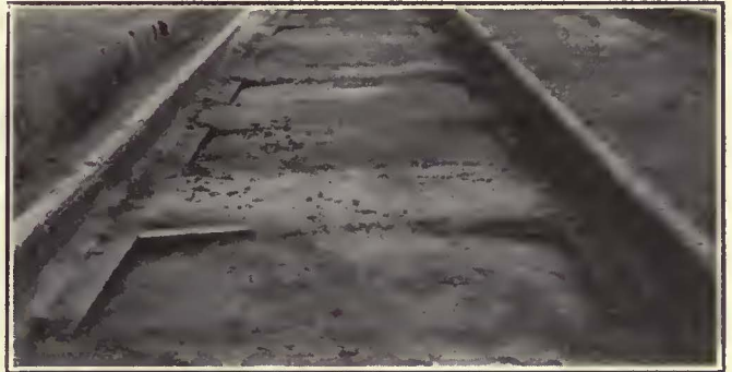
The Concrete Base Is Permitted to Set in This Form for Two or Three Days
