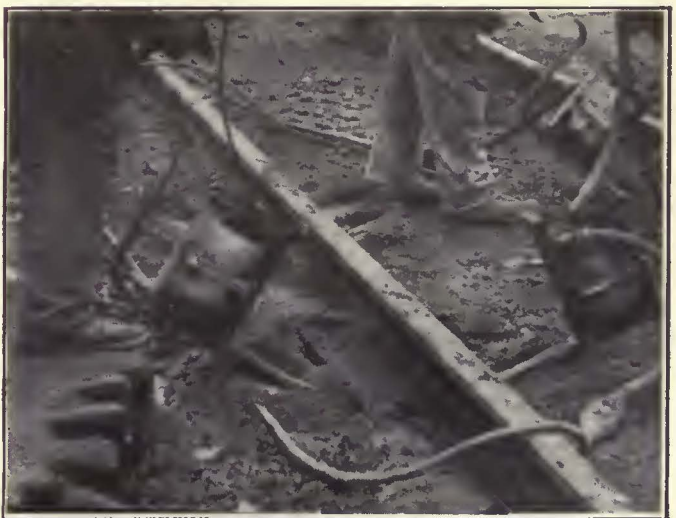
Closer View of Electric Tamping Tools Working Special Bearing Mix Under the Tie Plates
