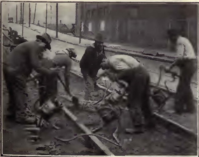
Pouring the Concrete Track Base and Leaving Openings Under the Tie Plates
