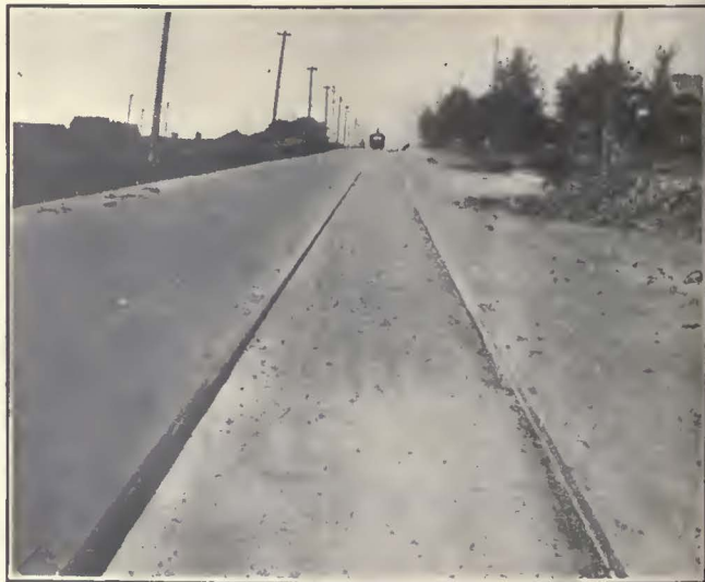
This Concrete Paving Between the Rails in Fort Worth Cost Only Half as Much as the Paving Elsewhere on the Street
