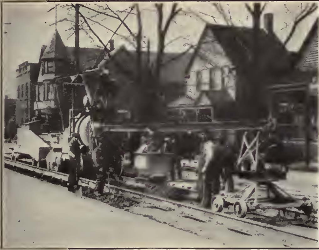
Pouring the Concrete Track Base and Leaving Openings Under the Tie Plates
