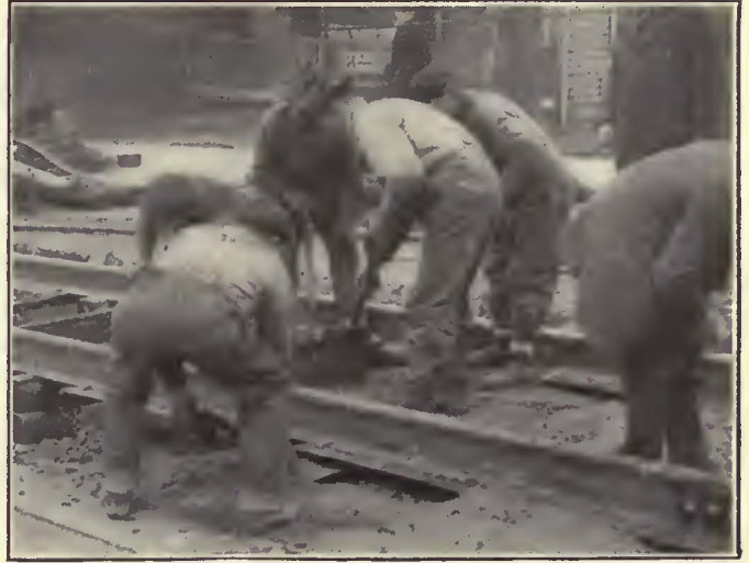
How the Concrete Is Distributed and the Under-Tie Openings Made with Shovels
