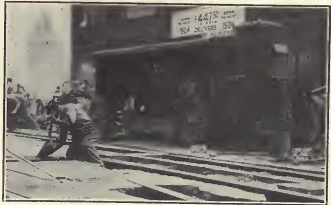
A 350-Cu.Ft. Compressor Was Employed to Expedite Track Reconstruction Work on Upper Broadway, New York
