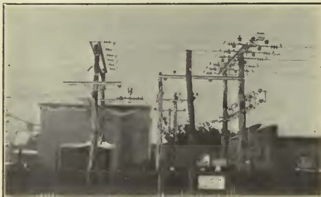
Front and Side of New Semi-Automatic Substation at Concord, N. H.
