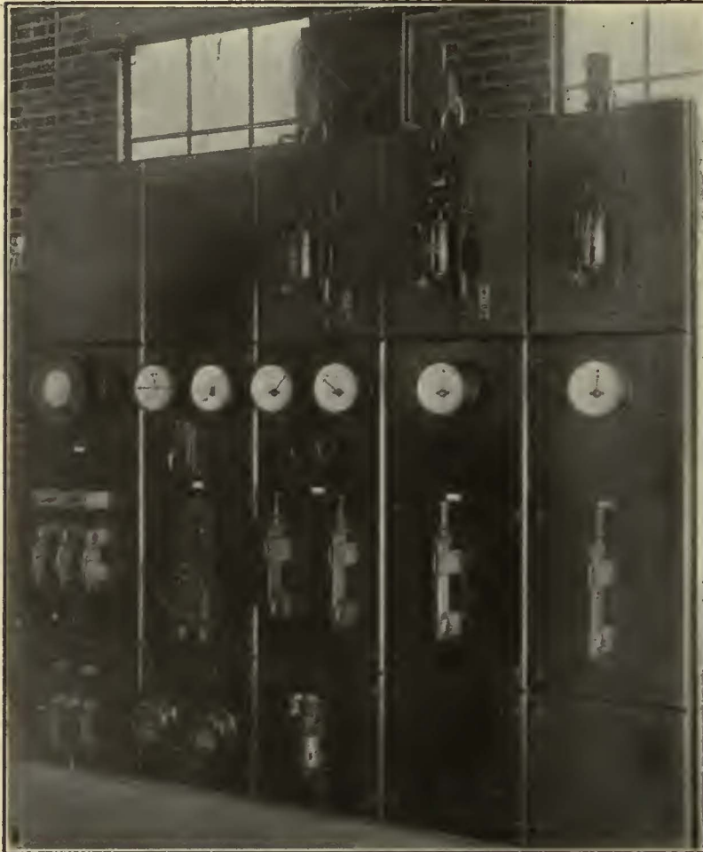
No. 1. The automatic switching equipment is shown at the tops of the switchboard panels.
