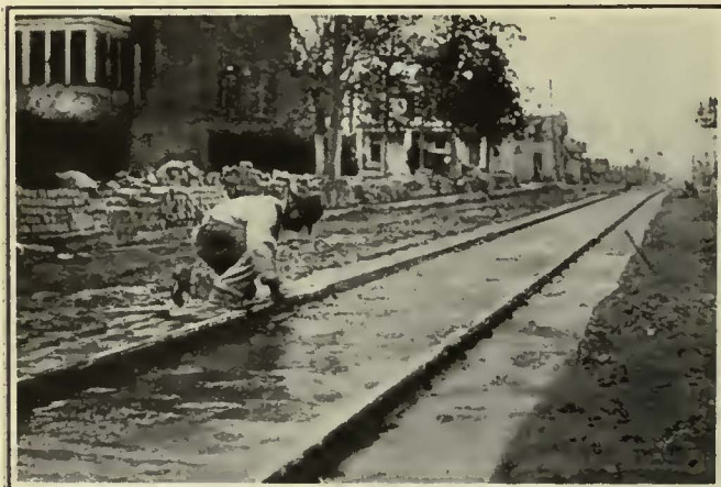
This Wet Mixture Is Used by the Northern Texas Traction Company Preparatory to Laying a Brick Pavement
