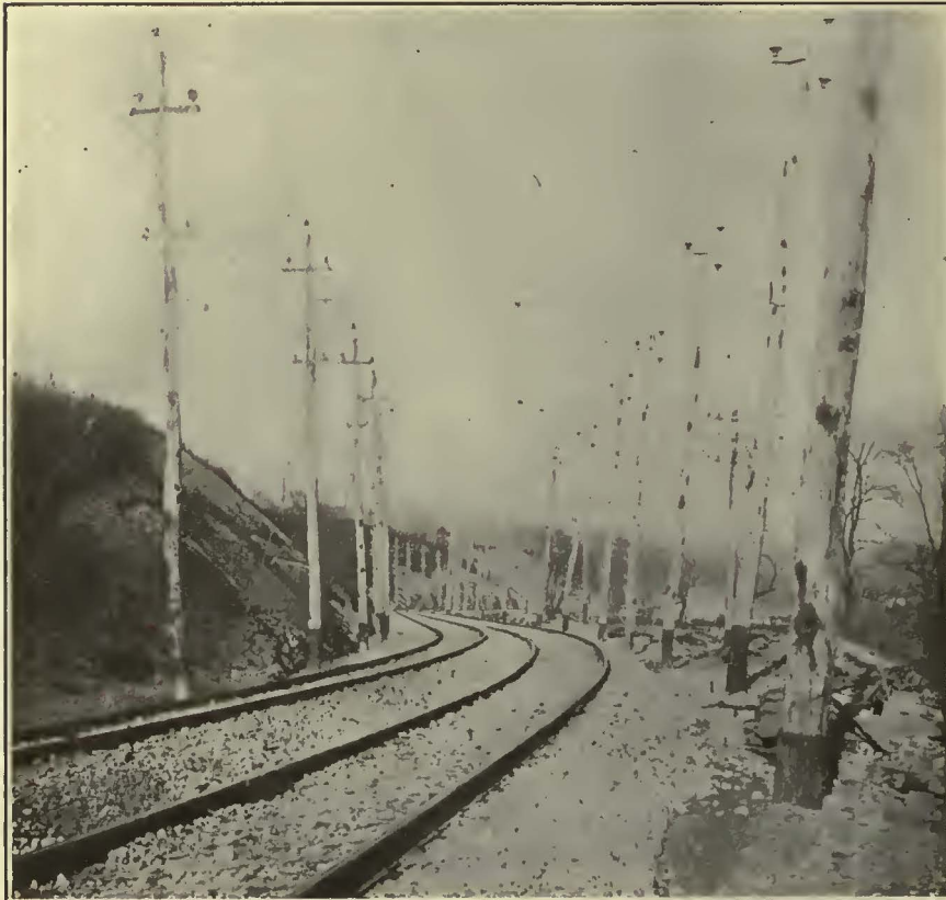
Typical Wood Pole Construction on Private Right-of-Way, Showing High-Tension, Feeder and Span Construction on the Same Pole Line
