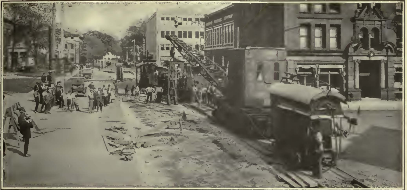
Large Air Compressor, Locomotive Crane, Air-Operated Pile Driver for Breaking Pavement, Work Car and Electric Shovel in Use in Reconstruction of Track on Onelda Street in the Center of Milwaukee
