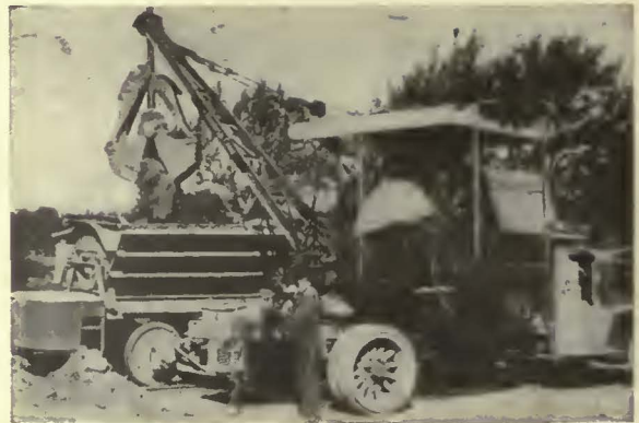
This machine sets poles, lays track or handles 200 to 300 yards of material a day for the Cleveland Railway Company.
