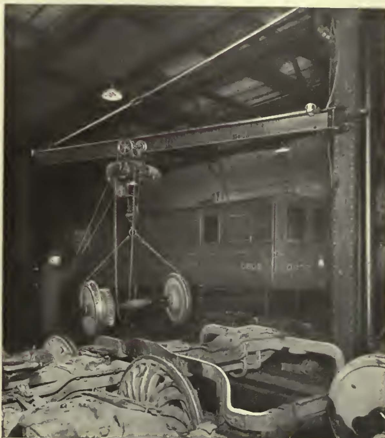
Electric Hoist on a 10-In. Swinging I-Beam, in the Shops of the Worcester Consolidated Street Railway. Motors, Wheels and Trucks Can Easily Be Moved from One Track to Another with This Apparatus
