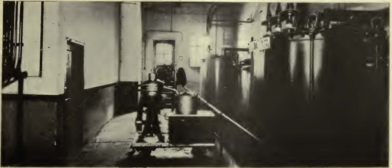
De Laval Transformer Oil Purifier in the West Tulsa Station of the Oklahoma Power Company.
