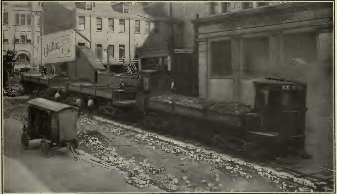
Differential Dump Cars Used in This Case to Haul Away from the Job Removed Paving Loaded by Electric Shovel
