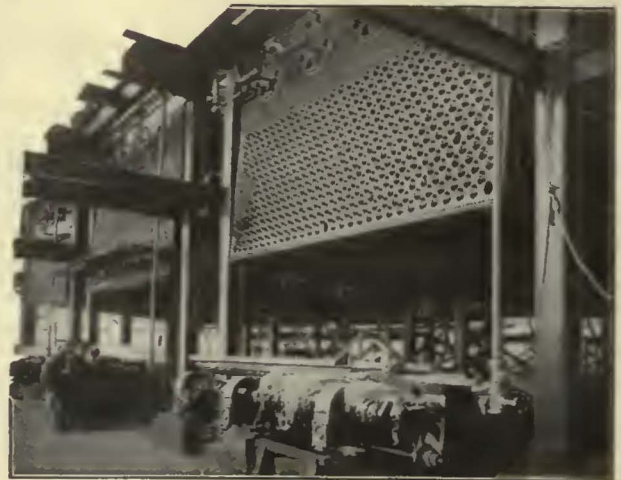
Below are shown three 1049 H. P. Edge Moor Boilers during erection at Westport.
