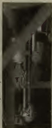
50 KV. Oil Circuit Breaker Contact Details Showing Contacts Completely Open.
