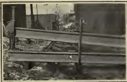
The Collar Is Placed Around the Joint to Be Raised and Pressure Applied by Means of the Jack
