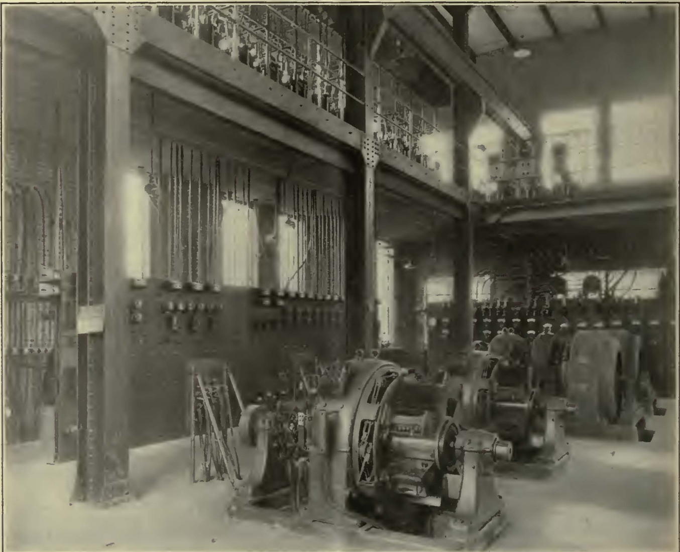
Rotary Converters and Motor Generators in Elgin Substation. Alternating-Current Switches Have Been Mounted on Balcony, with A.C. and D.C. Switchboards Below
