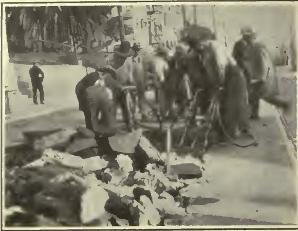
Pneumatic Paving Cutters Opening Up Pavement of 6-In. Concrete Overlaid with 3-In. Asphalt
