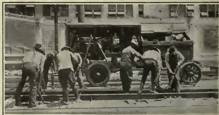
This Gas-Operated Compressor Used for Heavy Track Reconstruction Supplies Air for Eight Pneumatic Tools
