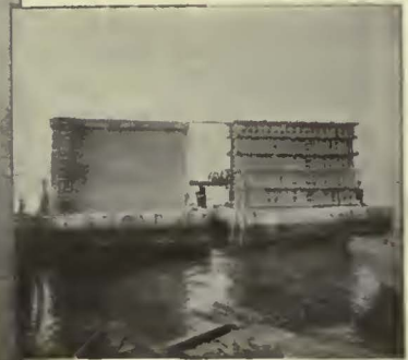
New structure is to be 7500 feet long with Concrete Piers weighing 1500 tons each.
