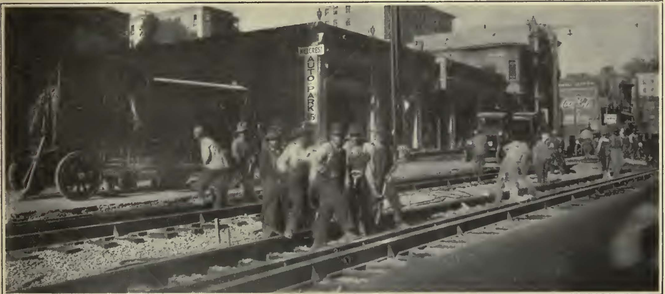
Three Air Compressors at Work Simultaneously in the Downtown District on Combination Gage Tracks, Where the Job Had to Be Done Without Interrupting a Thirty-second Headway
