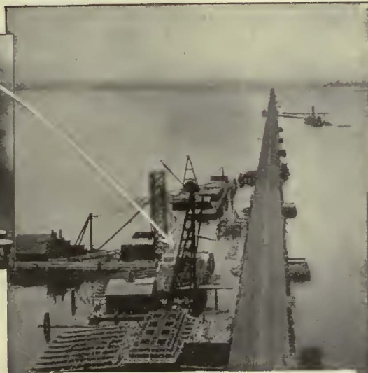
The new, four-track Central Railroad of New Jersey Bridge over Newark Bay will be located 100 feet north of the present structure. The new track level will be 30 feet higher than the old.
