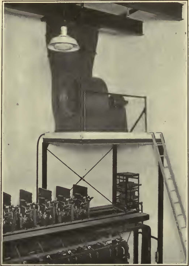
In the Fifty-fourth Street Substation the Exhaust Blower Is Mounted Above the Switchboard
