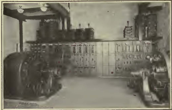
The Machine Room of the Two-Unit Melrose Substation. The Air Outlets Are Above the Grid Resistors
