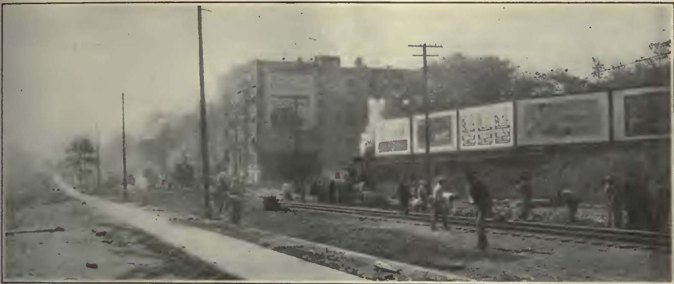
Careful Planning Made Possible the Completion of This Job in a Short Time. The Steam Shovel, Steam Roller, Track Layers, Joint Welders, Grinders, and the Paving Gang Followed One Another in Close Order
