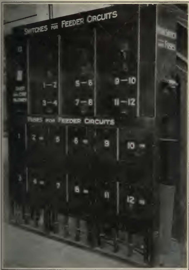
Switchboard for Feeder Circuits, with Fuses Inclosed in Cabinets Beneath
