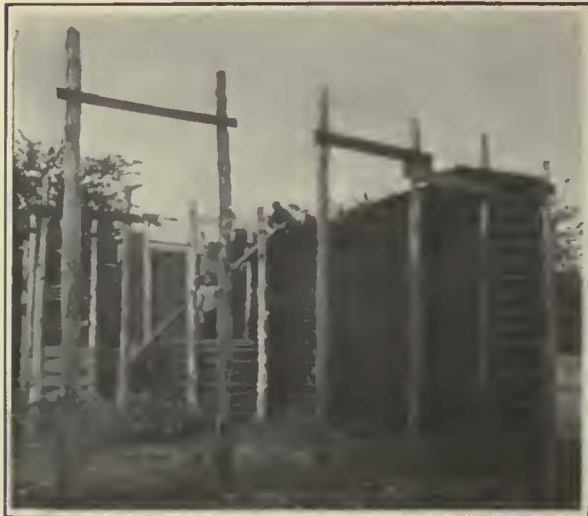
Fiber Conduit Is Stacked in Open-Air Racks. These Are Made of 12-Ft. Cedar Posts Having the Tops Tied Together with Guy Wire
