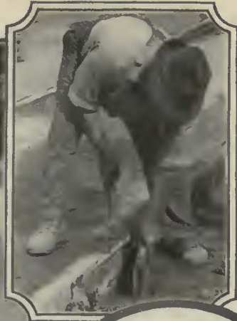
Installing Carey Elastite Rail Filler. A tap of the mallet sets it securely in place.
