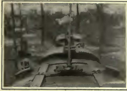
Trolley Base Is Supported on Flat Steel Bars Between Wood Strips 4 Ft. Apart
