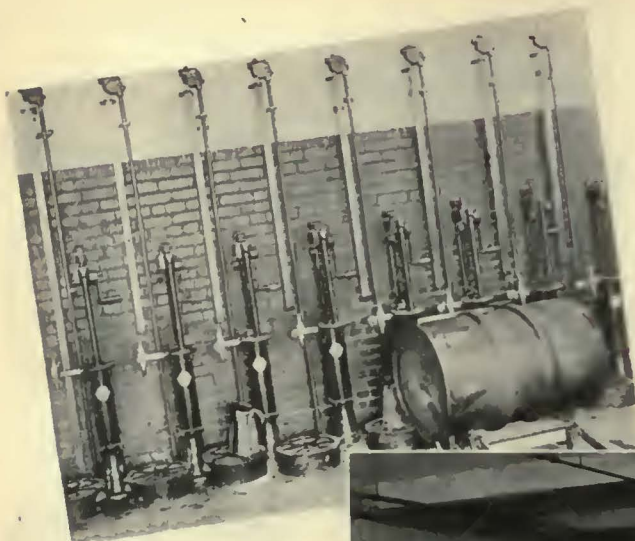
Battery of Self-Measuring Pumps Which Are Connected with the Basement Tanks. In the Foreground Is a Drum in Position for Emptying Into One of the Tanks
