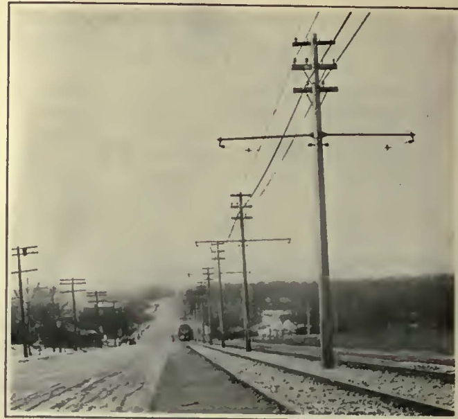
Concrete Poles of This Type Are Being Installed at the Rate of Approximately 100 per Year
