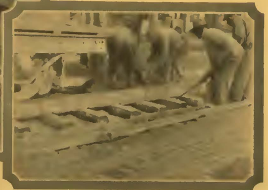
Below—Carey System of Track Insulation installed in Maryland Street tracks, Indianapolis, Ind.
