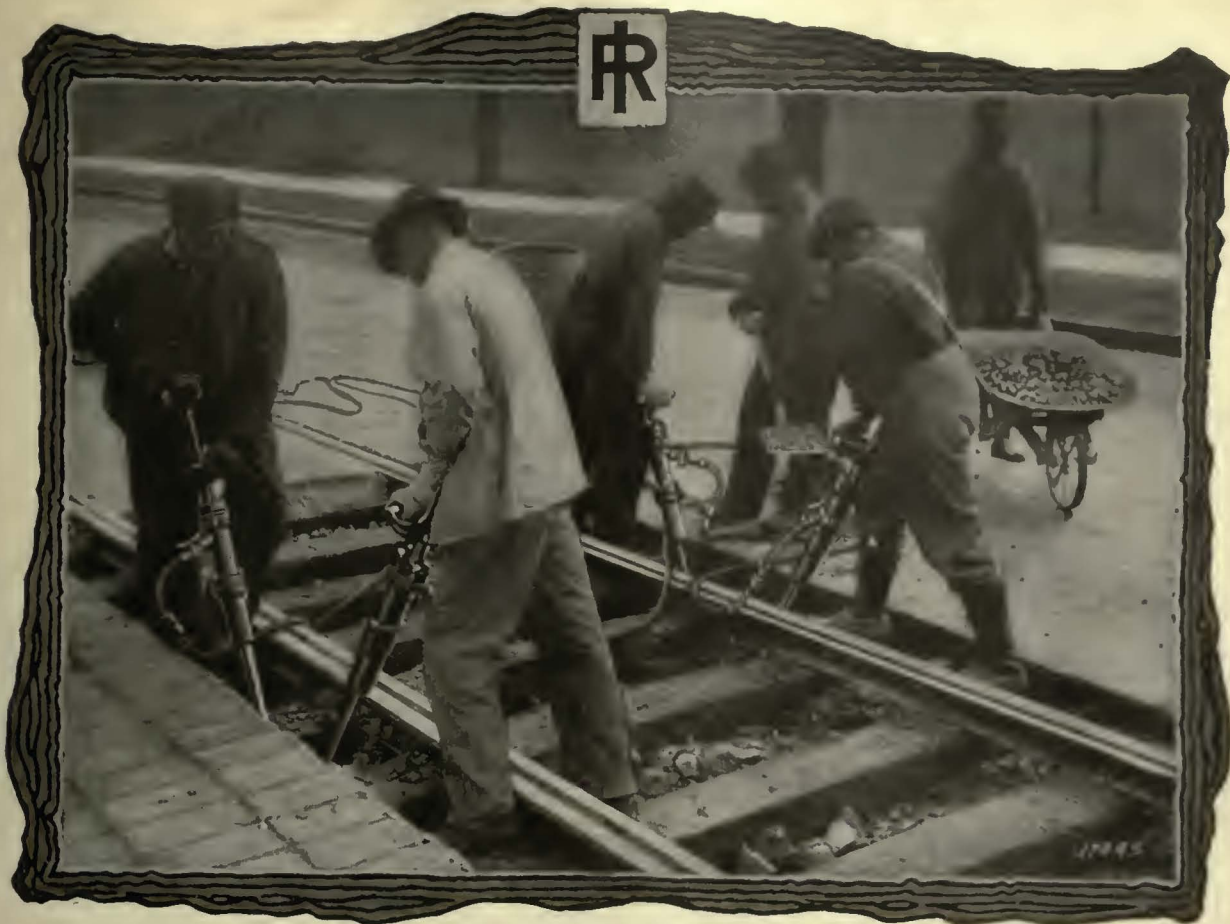
A four-tool pneumatic tamping gang at work on a track repair job
