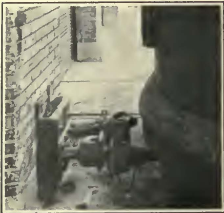
A Rack Mounted on a Carhouse Pillar Between Tracks Contains Two Types of Drawbars to Which a Car on the Transfer Table May Be Coupled for Testing the Coupler and Draft Rigging
