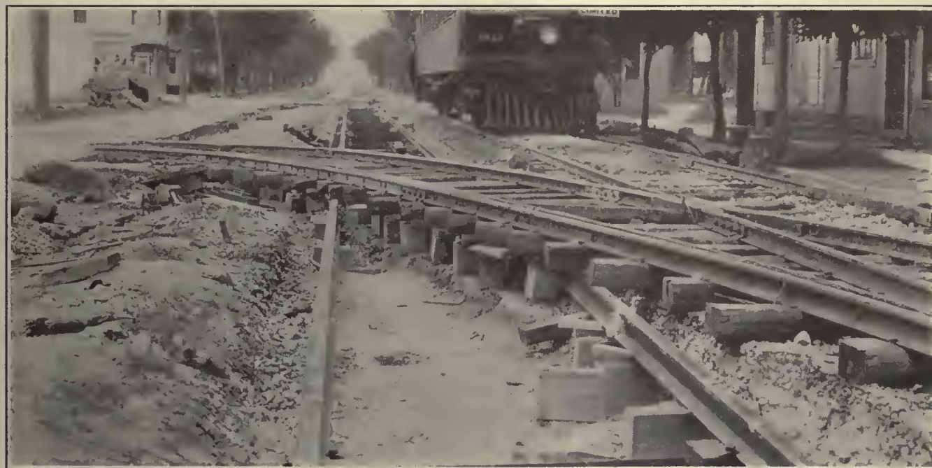
Temporary Crossing of Branch Line During Reconstruction Work at Sheboygan, Wis., Used While Rebuilding Main Line Tracks on Eighth Street
