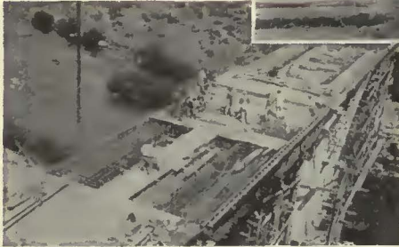
Construction Work—Bridge across Truckee River and S.P.R.R. tracks lo- cated in Nevada County, near Polaris.
