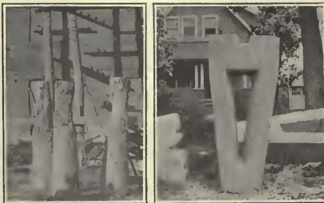
At Left, Decayed Butts of Old Poles Being Removed. At Right, Concrete Base Installed Under Old Poles
