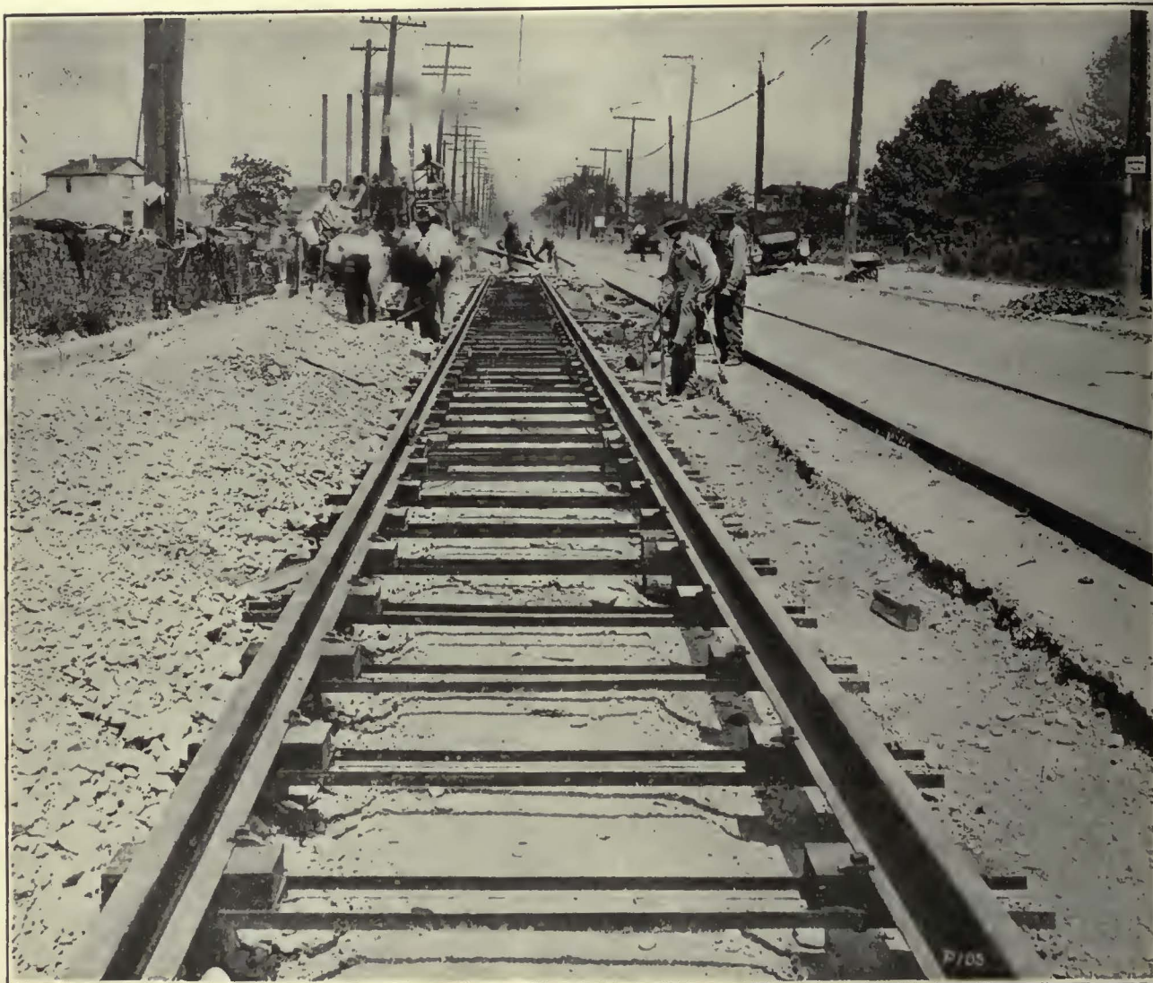
Troy Pike, Dayton, Ohio, when Dayton Ties were being put in under the southbound track of the Dayton & Troy Electric Railway.
