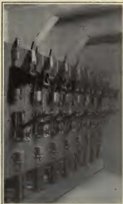
Front View of Group of Circuit Breakers in Chamber at 79th Street and Lexington Avenue
