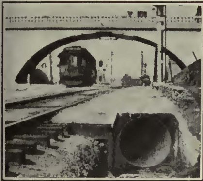
Corrugated Iron Culvert Installed Under Passenger Landing at Vinyard Station of the Pacific Electric Railway
