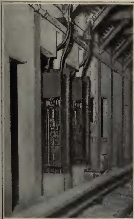
Circuit Breakers in Boxes on Columns, with Boxes Open at 136th Street and Alexander Avenue
