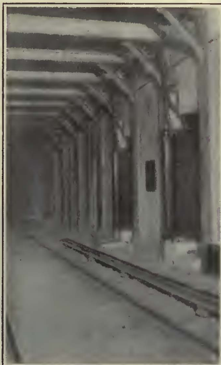
Circuit Breakers in Boxes on Columns with Boxes Closed at 129th Street and Lexington Avenue
