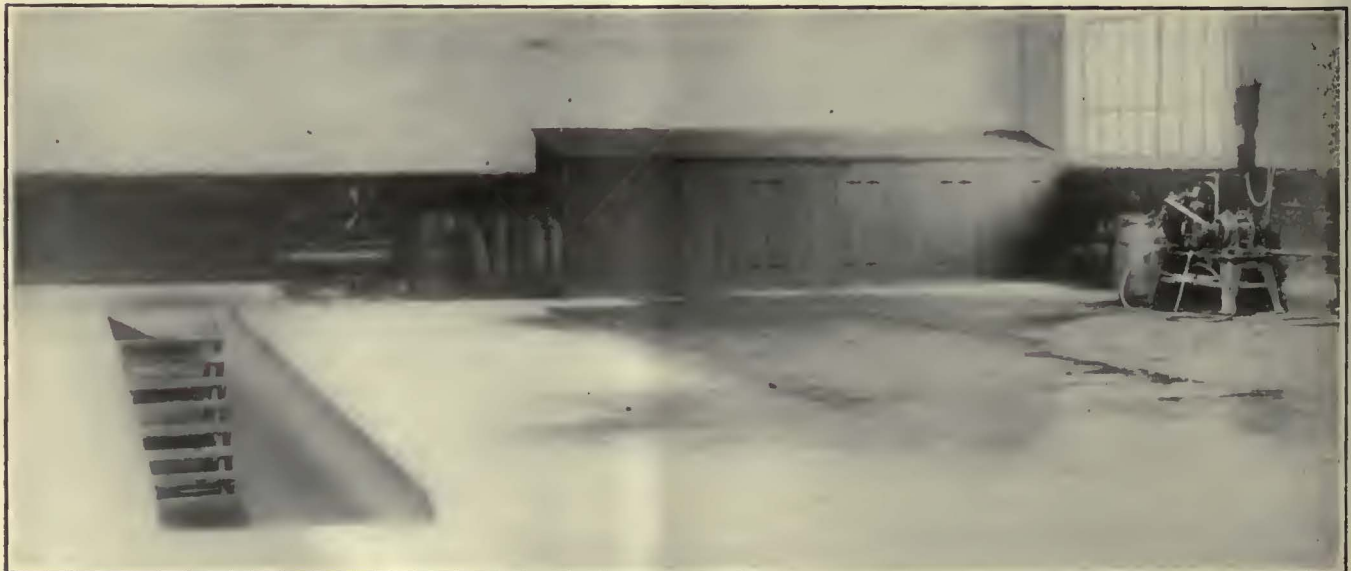
An Electrically Operated Spray Washer and a Portable Air Compressor Form Parts of the Equipment of the Bus Garage of the Dubuque Electric Company
