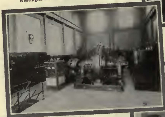
57th Street Substation Interborough Rapid Transit Co., New York Three 4,000 kw Westinghouse Synchronous Converters
