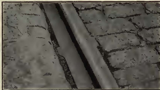
A Thermit Rail Weld made over 6 years ago in Grand Street, Jersey City, N. J.
