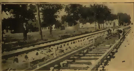
A view of the track system of the Wisconsin Power & Light Co. at Sheboygan, Wis. This shows the type of track construction together with the use of Carey Elastite Rail Filler which was being set in place when the photograph was taken.
