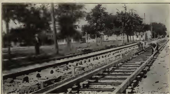
A view of the track system of the Wisconsin Power & Light Co. at Sheboygan, Wis. This shows the type of track construction together with the use of Carey Elastite Rail Filler which was being set in place when the photograph was taken.
