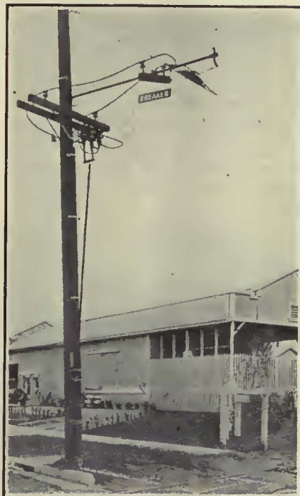
Combined Trolley Wire and Track Sectionalizing Switch in Open Position
