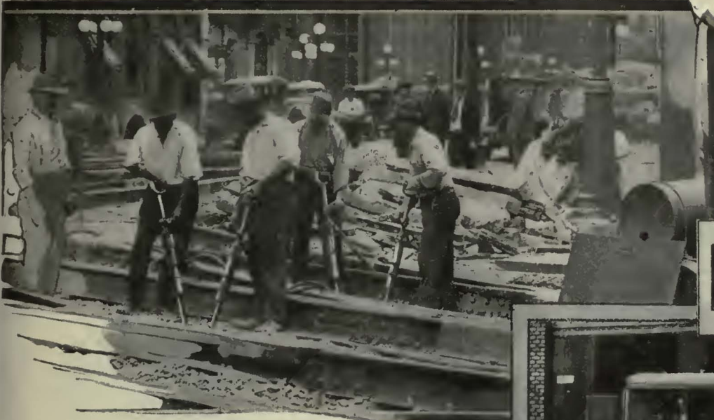
Center — Electric driven portable compressor supplies air for tie tampers or paving breakers.
