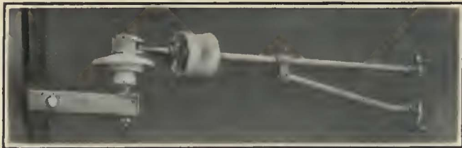
Hinged Bracket or Pull-Off as Used in the Section Equipped with Suspension Insulators
