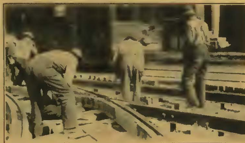
Fort Wayne electric railway tracks in process of construction—showing the slabs of Carey Elastite Rail Filler in place.
