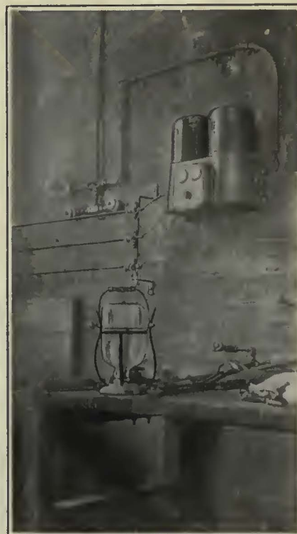
Wall Location of Battery Charger Economizes Shop Space
