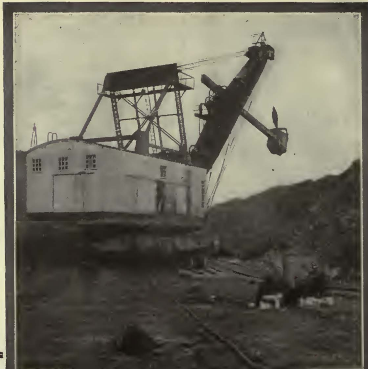
No. 4—3-conductor Super Service Cable—carrying 7500 volts to the big Marion Shovel, twenty-four hours a day.
