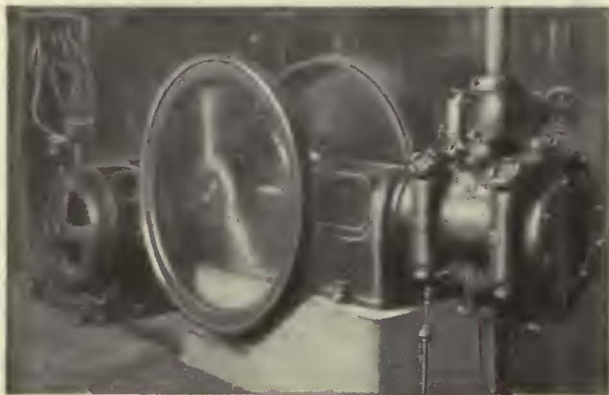
In this railway shop, the Sullivan "WG-6" Compressor supplies air by night, while the Sullivan Angle Compound Compressor in the background handles the heavier day demand.
