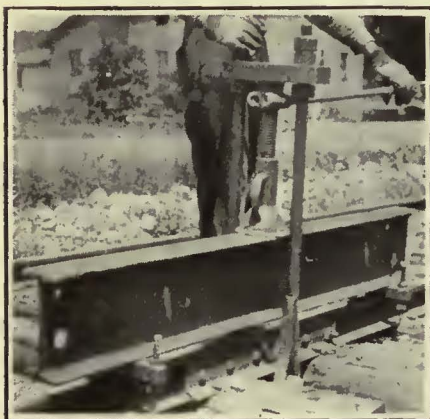
Screw Jack Exerts 15 Tons Pressure to Straighten Low Joints on T. H., I. & E. Lines
