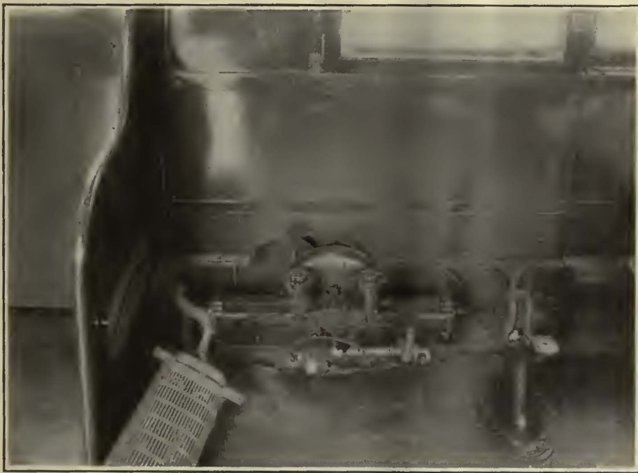
A New Type of Door Engine Is Being Installed in the Door Pocket
