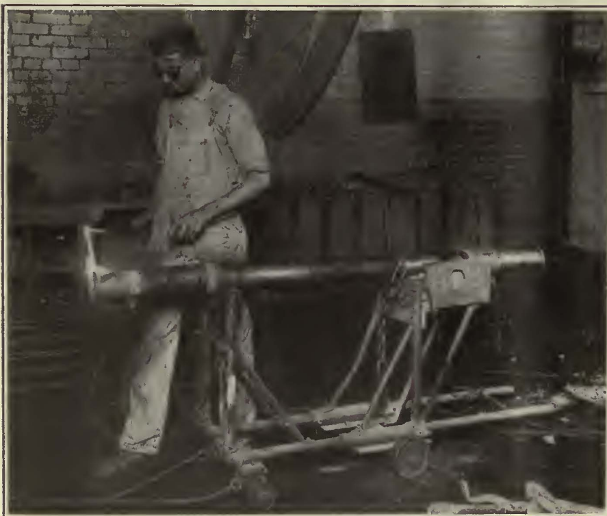
Dallas Railway Builds Up Car Axles by Welding Process. Note the Handy Buggy Constructed Out of Pipes and Fittings
