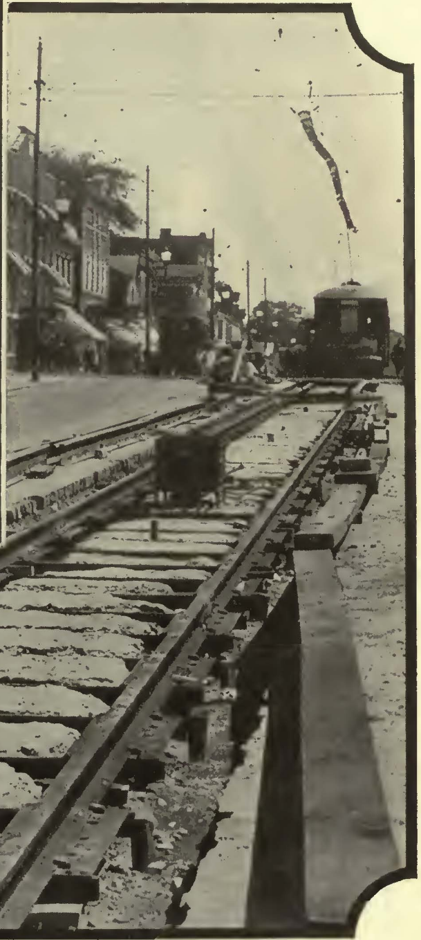
Renewal on old base—Bridge St., Oswego, N. Y. The Empire State Railroad Corporation
